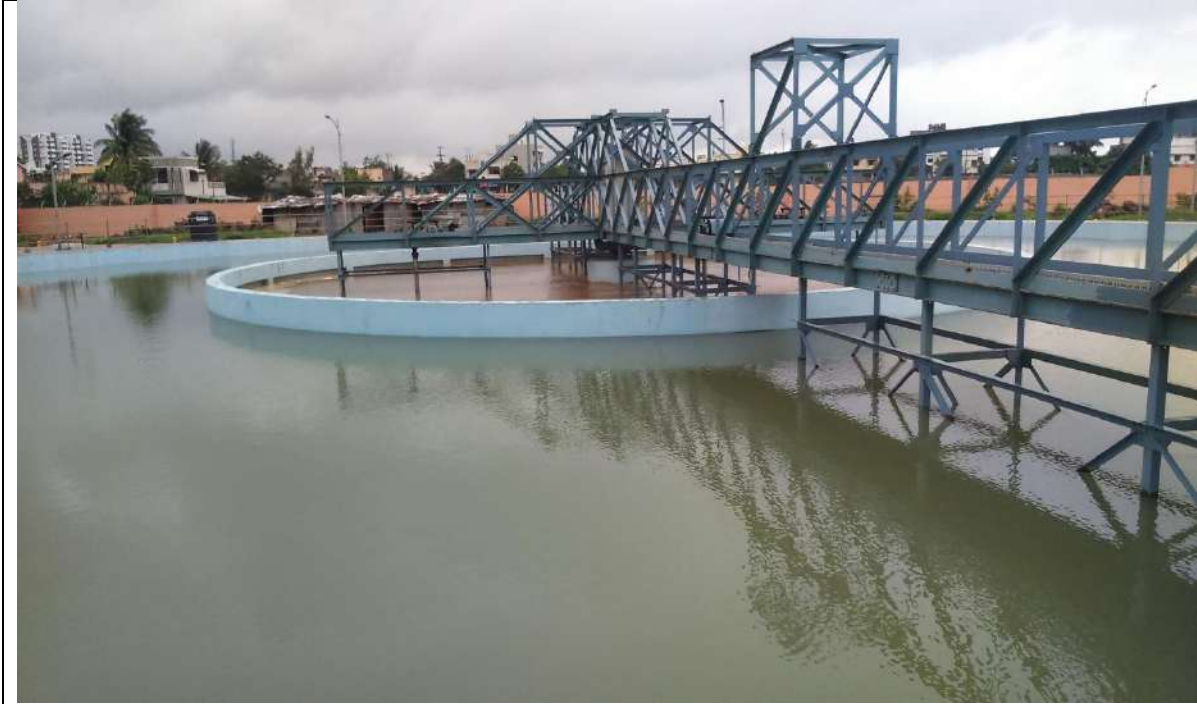
Nilgiriabaugh Water treatment plant: Clariflocculator
