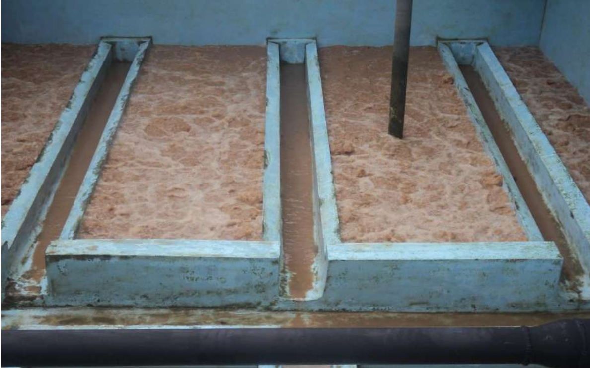
Back washing of Rapid Sand Filters
