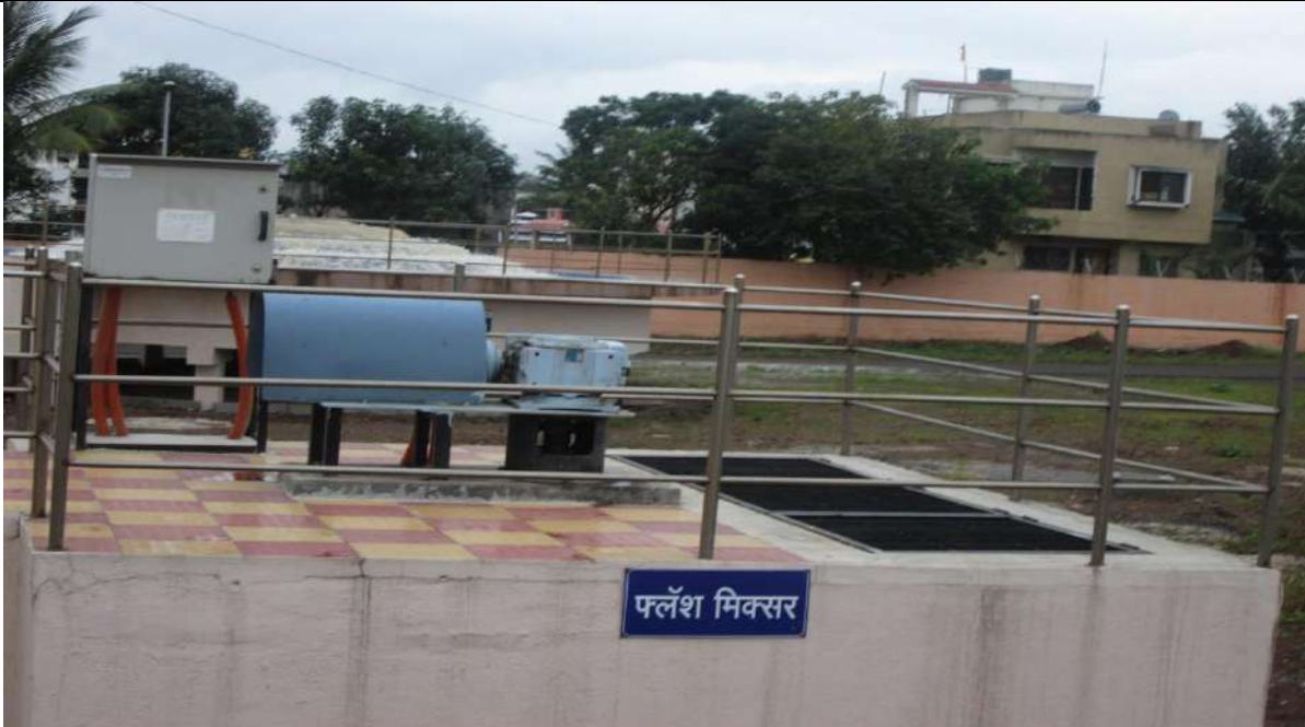
Flash Mixer at Water treatment plant
